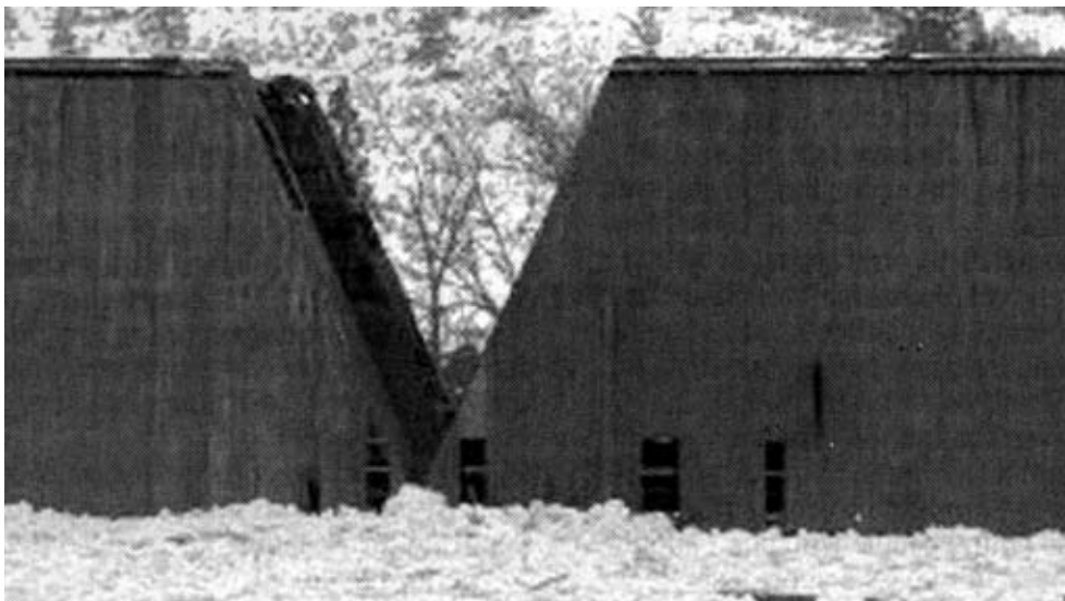
The Red Bridge over the Similkameen River west of Keremeos was reopened to traffic Thursday, one day after being threatened by a massive ice jam that flooded nearby properties. At least 20 properties suffered damage.
